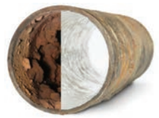
New cast iron pipe vs. buildup in cast iron pipe
